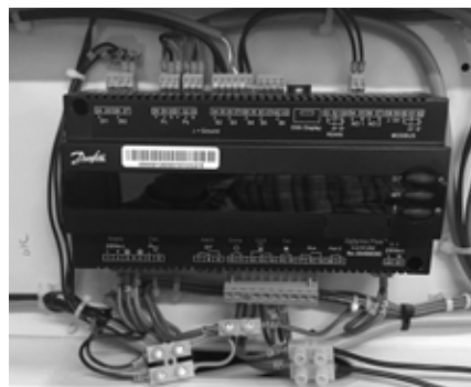
Picture 4 : Temporary wiring
