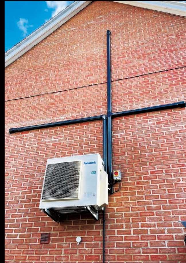
ADL Air Conditioning (UK)
